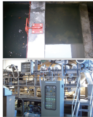
Installation of Oil-Water Separator Replacement of wornout dehydrator at the wastewater treatment plant of Daejeon Plant
